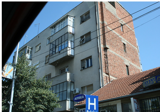
FIGURE 25: Unfinished buildings in urban areas (photo by C. Potsiou)
